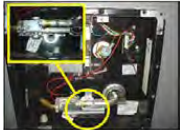
Fig 1: Water heater drain plug
