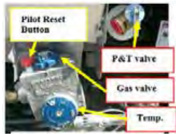
Water Heater pilot ignition
