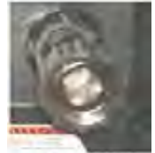
Fresh water inlet valve
