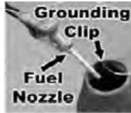
Fuel Nozzle in contact with receiving tank
