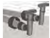
Low Point Drains
